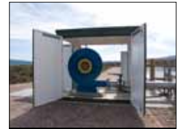
Low pressure, low energy fan blowers require little maintenance and only run when required by loading.
