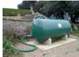
Septage reception station for insertion of locally collected septic tanks into the Accel-o-Fac system.
