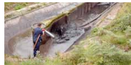
Sludge and peak flows from the existing ditch are diverted to the Aero-Fac® Sludge Digestion System.
